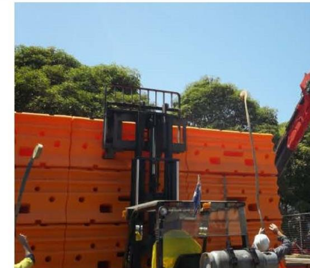
All layers must be individually strapped. The forklift must remain still to protect workers until restraints are applied. Without stanchions the top layer may need to have 1 less row.
